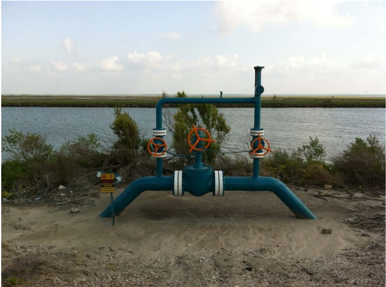
Figure 40. Enterprise pipeline service outlet believed to have been the source of elevated methane and TNMHC in March 2012.
